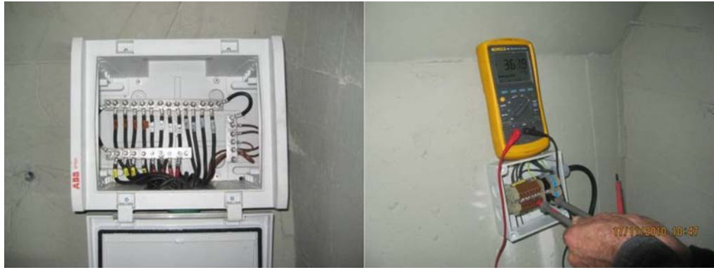
Figure 9. Detail of a connection box and the procedure of measurement of the voltage.
