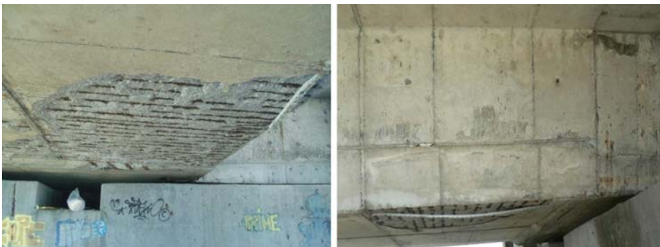
Figure 5. Affected areas of the bottom of the concrete girder.
