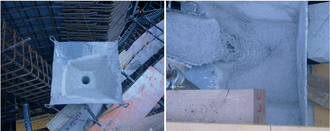
Figura 30. Hormigonado de los muros (a y b). Fuente ATESEF Figure 30. a) and b). Placement of concrete in walls. Source: ATESEF
