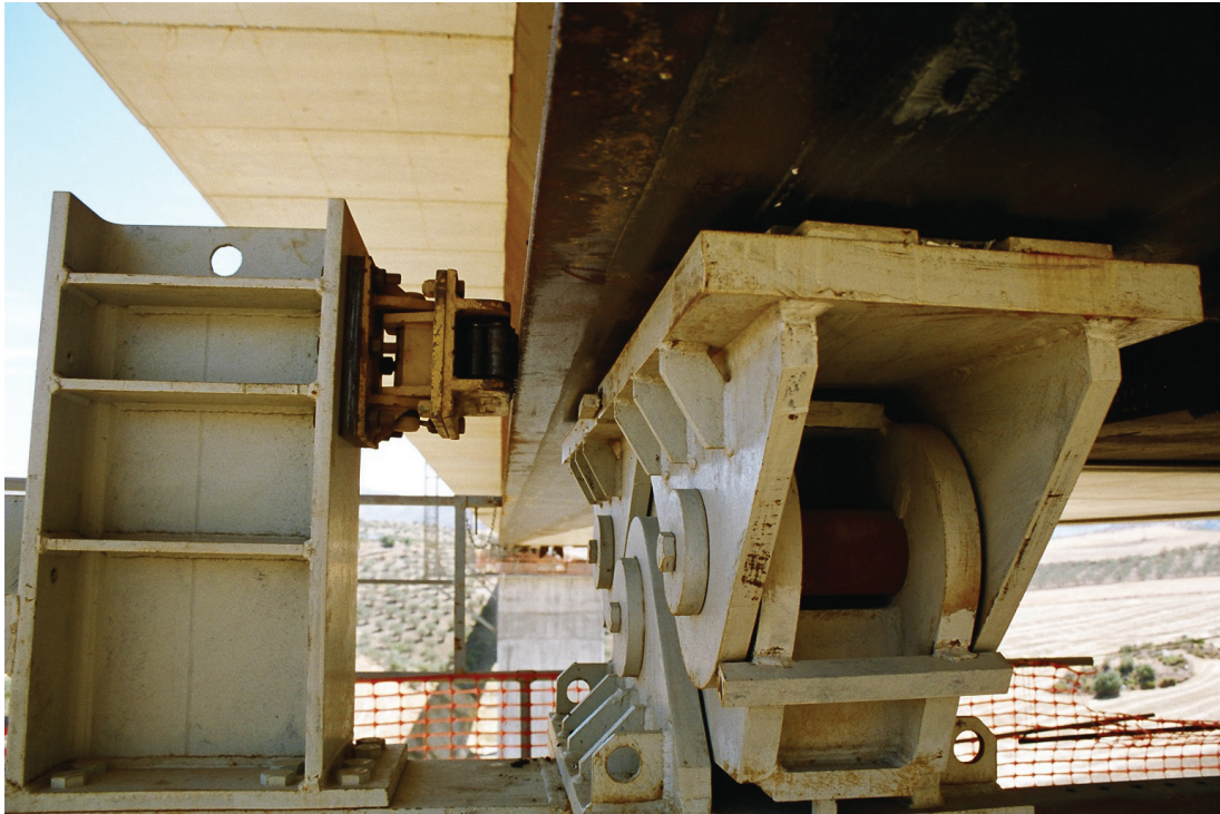
Fig. 18. Detalle de apoyos deslizantes con topes laterales durante el empuje. Fig. 18. Detail of sliding bearings with side stops during launching.
