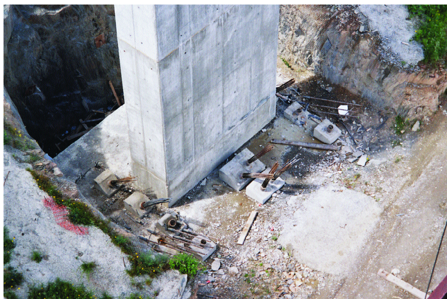
Fig.31. Anclaje de pila 8 al terreno. Fig.31. Anchoring of pier 8 to the ground.
