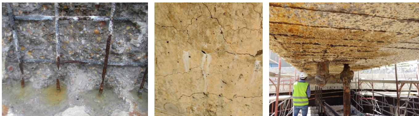
Figure 8. Different causes of deterioration of reinforced concrete: pitting corrosion (left), AAR (centre), acid attacks (right).
