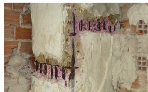
Figure 7. Example of a column where the carbonate concrete has reached the position of the rebars.
