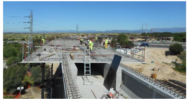
Figure 36. Construction of top slab by means of thin precast slabs over precast U beam
