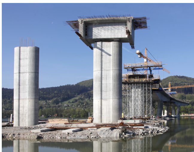
Figure 16. Deck of the approach spans of the Bridge across the River Vah's Reservoir.
