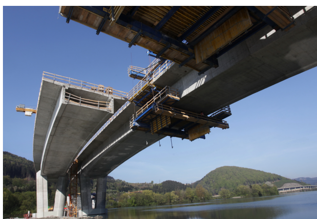
Figure 15. Deck of the main spans of the Bridge across the River Vah's Reservoir.
