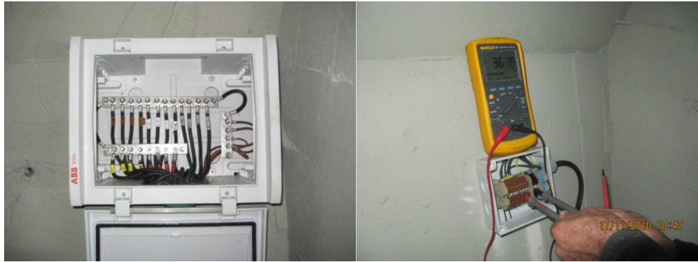
Figure 9. Detail of a connection box and the procedure of measurement of the voltage.
