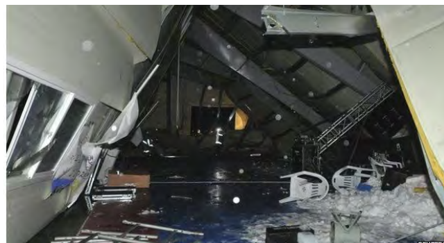
Figura 2. Collapsed frame-type roof structure with life-saving spaces inside the building [25].
