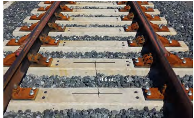
Figure 1. Usual distance between sleepers in Europe 0.6 m in High Speed and conventional ballast track.
