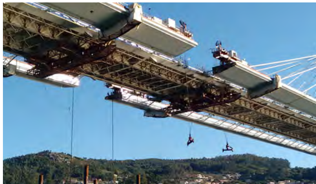
Figure 2. General view of the bridge during the closing with lifting of the penultimate segment.
