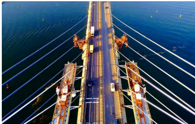
Figure 1. Top vie of the bridge from the other pier during an intermediate phase of the widening.
