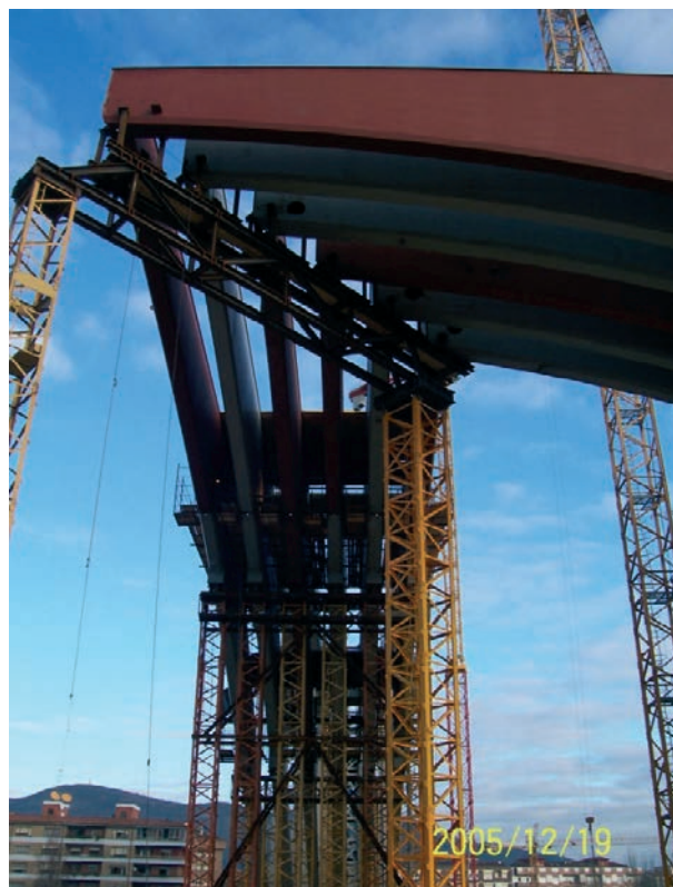
Figura 44. Torres de apeo con celosía superior en las intersecciones Sur-Este y Sur-Oeste Figure 44. Auxiliary supports with upper truss in the South-East and South-West intersections
