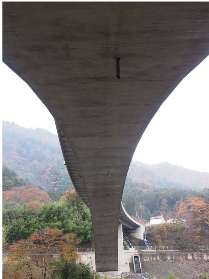
Figure 14 Deviation of arche and curved girder
