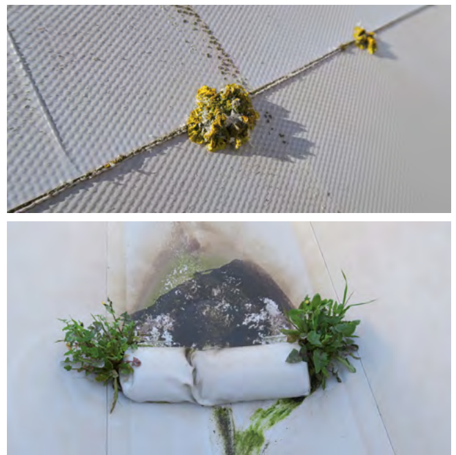
Figure 7. Some evidence in lack of maintenance. Credit: schlaich bergemann partner.
