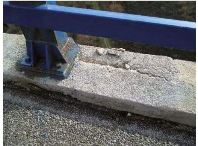
Figure 5. Detail of strapping damages.
