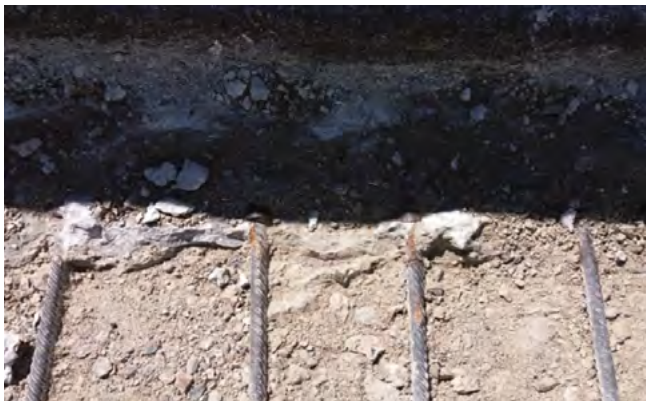
Figure 23. Detail of mechanical couplers.
