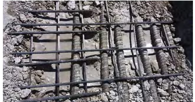
Figure 25. Post-tensioned sheath details with deterioration.
