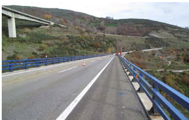
Figure 7. View of the state of the parapet (2015).
