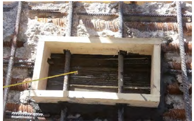
Figure 26. Deteriorated sheath sealing boxes.
