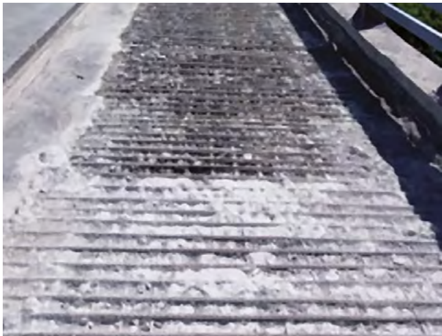
Figure 22. Existing reinforcement exposed.
