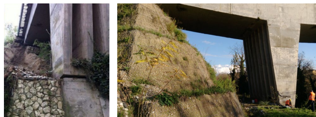
Figure 6. The landslide of the slope in 2015 and the armed lands behind the pier.
