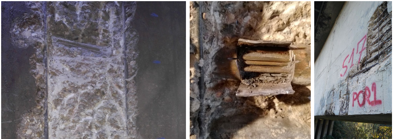
Figure 12. From the left: duct filled with mortar, duct not filled with mortar and degradation of the deck due to water.
